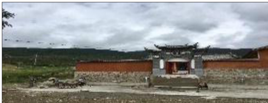
Figure 2: Temple to the Dragon King under construction. Our conversations with workers building the new Black Dragon King temple said they were paid 130 yuan a day (approximately $22.50). Volunteers also helped with the building. The workers revealed that their wages and the repairs overall were financed by people working outside the village.
